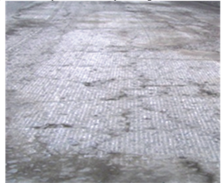
d) Cracks of corresponding base layer
