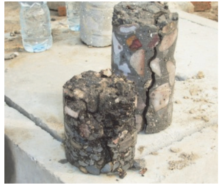
b) Core samples at corresponding transverse crack
