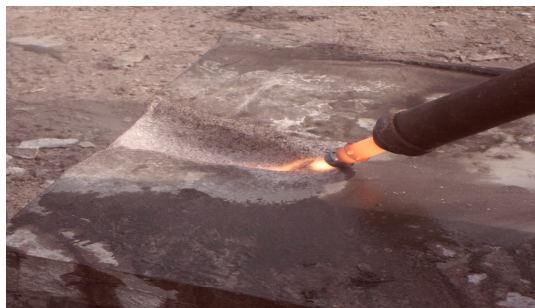
Fig. 5. Formation of slotted working by using BVR60 thermal cutter torch with gas-dynamic nozzle
