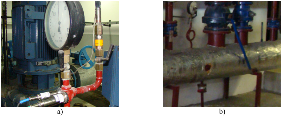
Fig. 12. Measuring points a) SBC placed close to working in systems pump, b) SBC located on transmission part of pipework
