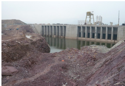
Fig. 2. The blasting site for rock excavation of open channel on land in Taishan
