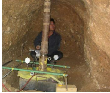
Fig. 2. In hole plate load test experiment to evaluate the in-situ elastic modulus
