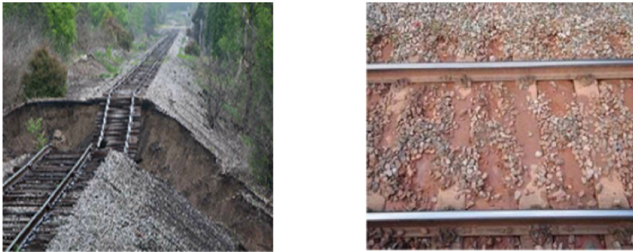
a) b) Fig. 1. Failures of: a) saturated railway embankment in 2011, b) mud pumping under dynamic train loads in UK
