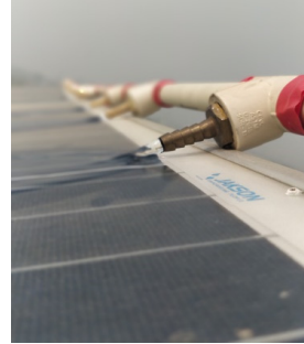
Fig. 4. Picture of nozzles for cleaning the PV modules
