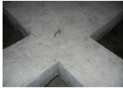
b) Cracks near frame beams
