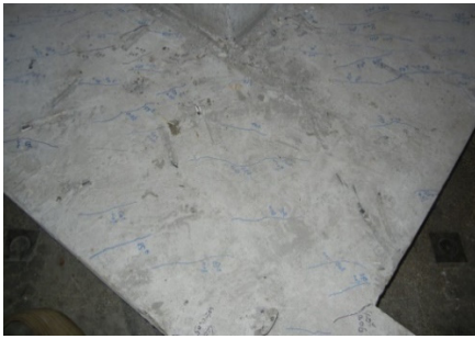
a) Cracks around corner of shear wall
