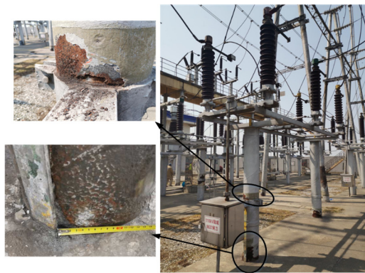
Fig. 1. Zhenyang 220kV substation's corroded steel columns
