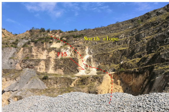
Fig. 2. F15 Exposed on the northern slope of the open pit. Photo by Wang Feifei, Sichuan, China, July 5, 2023
