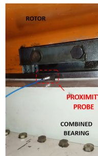
b) View of proximity probe and installed at 0° on combined bearing
