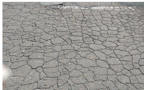
Fig. 4. A network of cracks. Photo was taken by Mamatkulov Muzaffar in October 2023, in highway D012
