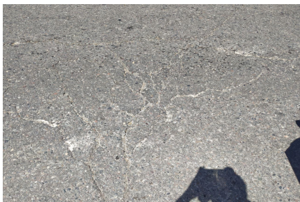
Fig. 3. Both transverse and longitudinal cracks. Photo was taken by Mamatkulov Muzaffar in October 2023, in highway D001
