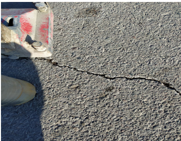
Fig. 1. Transverse cracks. Photo was taken by Mamatkulov Muzaffar in October 2023, in highway M39b
