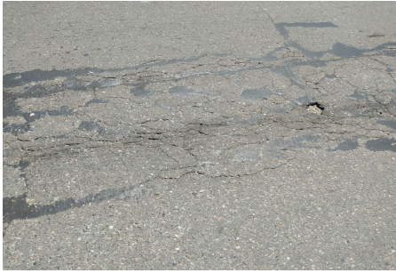
Fig. 5. The process of turning cracks into grooves. Photo was taken by Mamatkulov Muzaffar in October 2023, in highway D012
