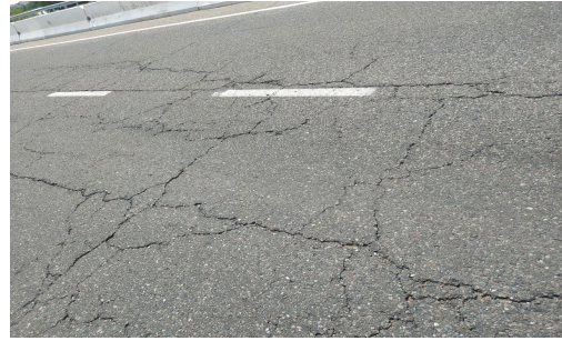
Fig. 6. Y and X-shaped cracks. Photo was taken by Mamatkulov Muzaffar in October 2023, in highway D021
