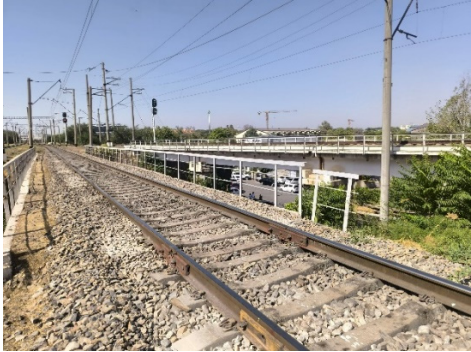
Fig. 1. In the transition section, increased vibration of the road's upper structure occurs due to the deformation of the embankment soil, leading to the crushing of ballast materials. The photograph taken by the second author on August 25, 2025, depicts the process of examining issues in the railway superstructure elements at the junction zone between the earthwork and the bridge
