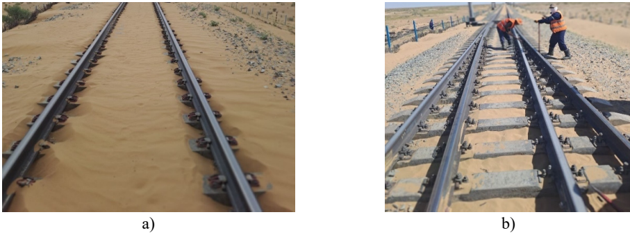
Fig. 7. a) Sand accumulation on the track superstructure; b) sand accumulation in a turnout (switch). Photos by A.Sh. Uralov, during field research conducted in April 2025 on the Bukhara-Miskin railway line (Qorlitog + -Kiyikli section)
