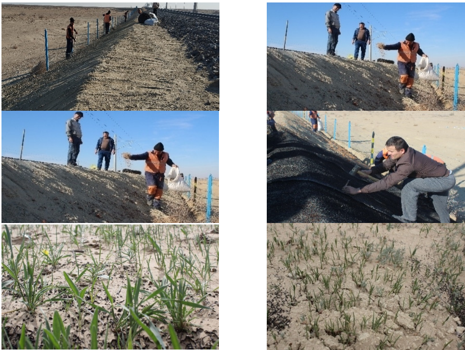
Fig. 9. Bukhara-Miskin railway line installation of anti-erosion geomat November 2024 and Observation results obtained in April 2025. Photos by A.Sh. Uralov, during field research conducted on the Bukhara-Miskin railway line (Qorlitog'-Kiyikli section) in November 2024 and April 2025
