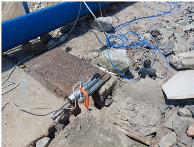
Fig. 4. Photo of the position transducer installed between the decks on top of the bridge. The photo was taken by S. Takhirov on May 30, 2025
