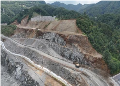
Fig. 4. Real scene of southern slope failure. Photo by Jia Haipeng in May 2024 on the south slope of the Longyu Large Open-Pit Mine
