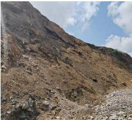
Fig. 13. Localized Landslide Map. Photo by Jia Haipeng in September 2025 on the south slope of the Longyu Large Open-Pit Mine
