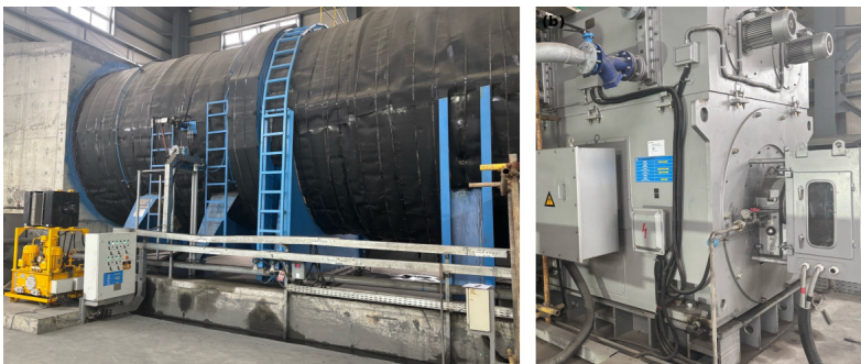
Fig. 1. Main mine ventilation fan and monitoring arrangement. Photo by the authors at Serbia Zijin Mining, 2025
