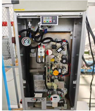
Fig. 3. Switch cabinet for experiment
