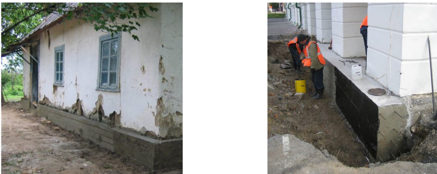
Fig. 1. Technical measures used to reduce soil salinization in the building area at the “Bog’don dalalari” farm, Pakhtakor district, Jizzakh region, Uzbekistan. Photos by the authors, 2024
