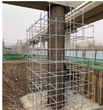
b) Arrangement of shear reinforcement and application of epoxy resin bonding agent
