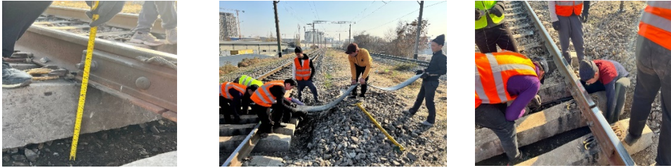
Fig. 2. Installation process of under-sleeper elastic pads in the rail joint zone. Photos by the second author on November 21, 2025, illustrate the process of experimental studies on the installation of elastic pads
