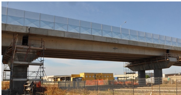
Fig. 1. Prestressed reinforced concrete viaduct representing the first case study. Photo by the authors during field investigation
